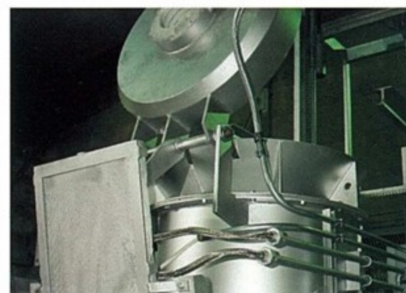
材料予熱室(タワー) Pre-Heating Tower
